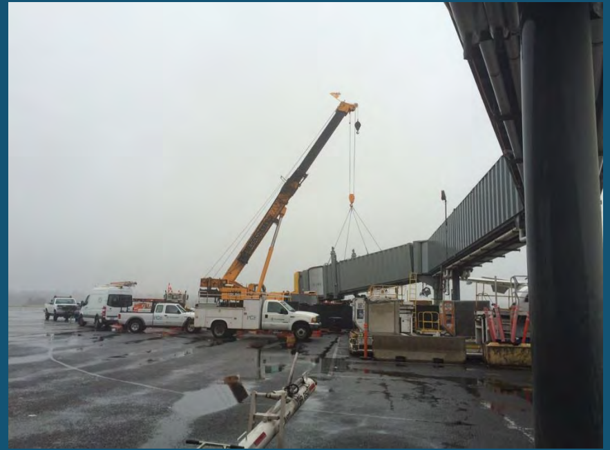
Passenger Loading Bridge – Gate S15
